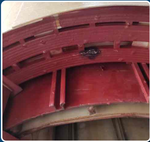
COIL INTER TURNS FAULT
