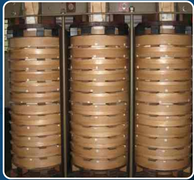
1500 KVA AFTER REWINDING
