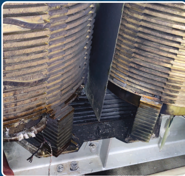
FLASHOVER BETWEEN COILS
