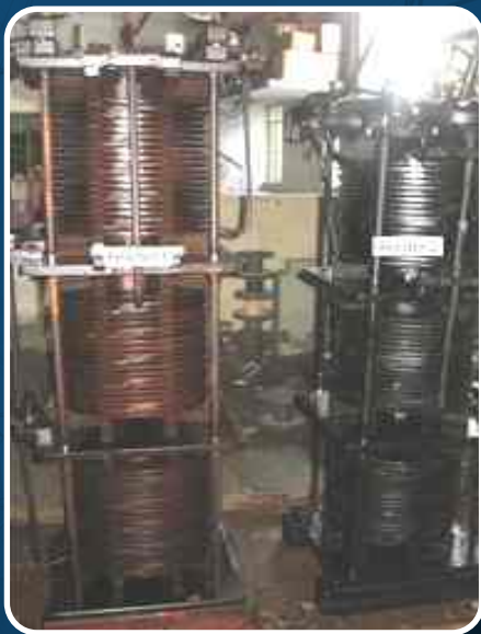
33 KV SERIES REACTOR
