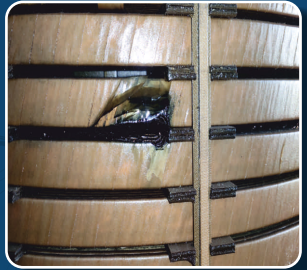
COIL INTER TURNS DAMAGE
