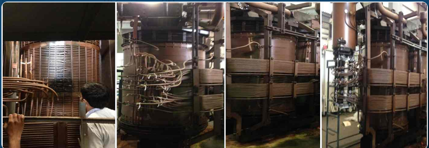
FAULT ANALYSIS OF 25 MVA TRANSFORMER
